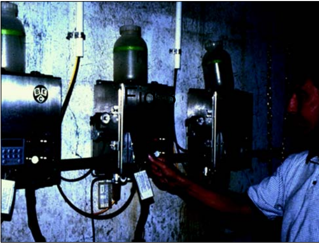
Assistant Plant Manager Doug Wise checks sampler cycle times, individually adjustable for each sample point. Panels actuate the Isolok samplers with compressed air for greater safety and direct air passes through the sampler bodies to help eject sluggish materials.
